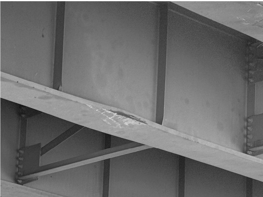
EXISTING GIRDER 3 IMPACT DAMAGE
